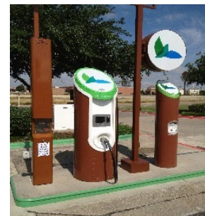
Curbside DC Fast Charging EVSE
