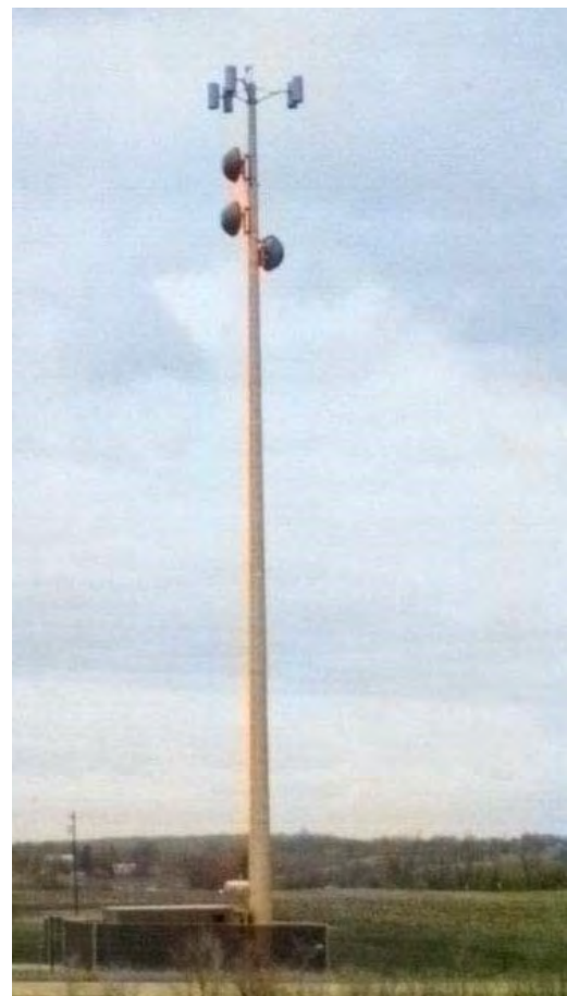
MONOPOLE TOWER (MOUNTED WITH DISHES)
