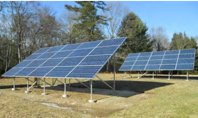
GROUND MOUNT SOLAR
