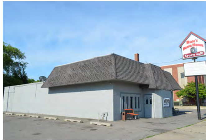
4 GRADE CONCRETE BLOCK – WOOD FRAME
