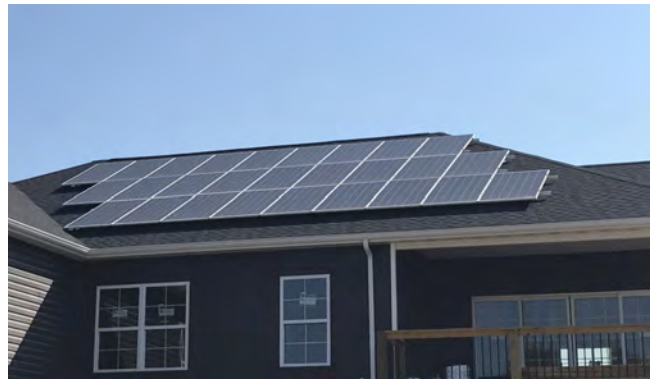
ROOF MOUNT SOLAR
