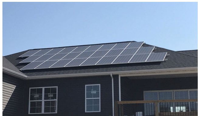
ROOF MOUNT SOLAR
