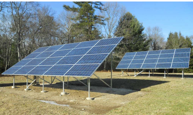
GROUND MOUNT SOLAR
